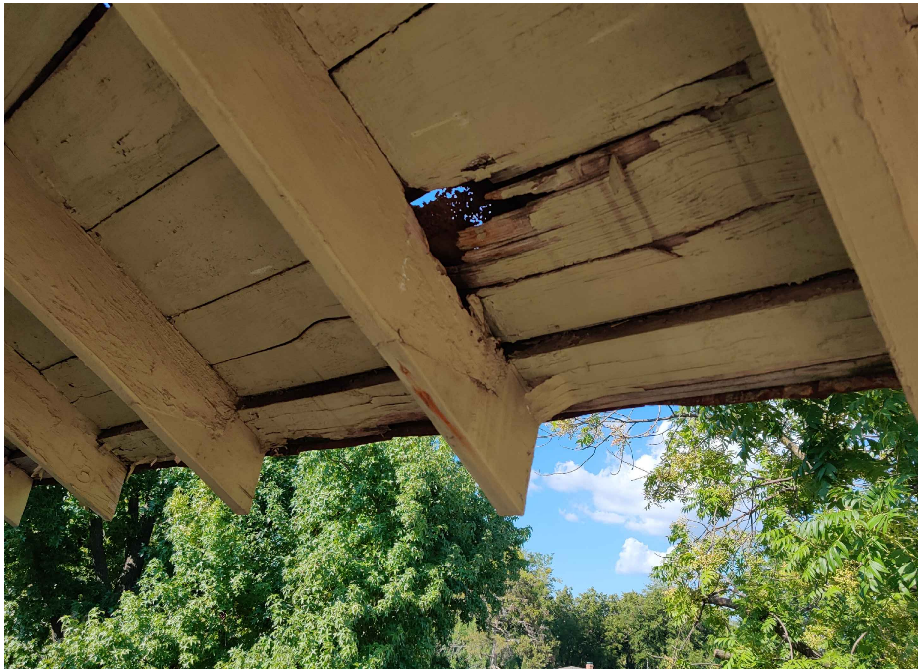
PHOTO- FAILURE OF ROOF AND DECK
