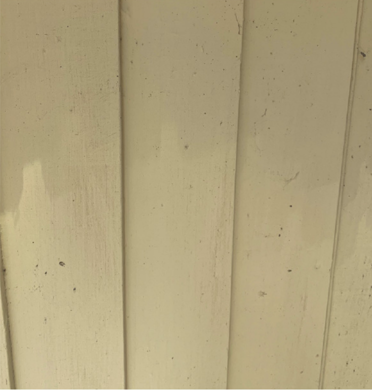
EXISTING 4 1/2" H. WOOD LAP SIDING TO BE REMOVED AND REINSTALLED NEW WOOD LAP SIDING TO BE MILLED TO MATCH EXISTING AS REQUIRED
