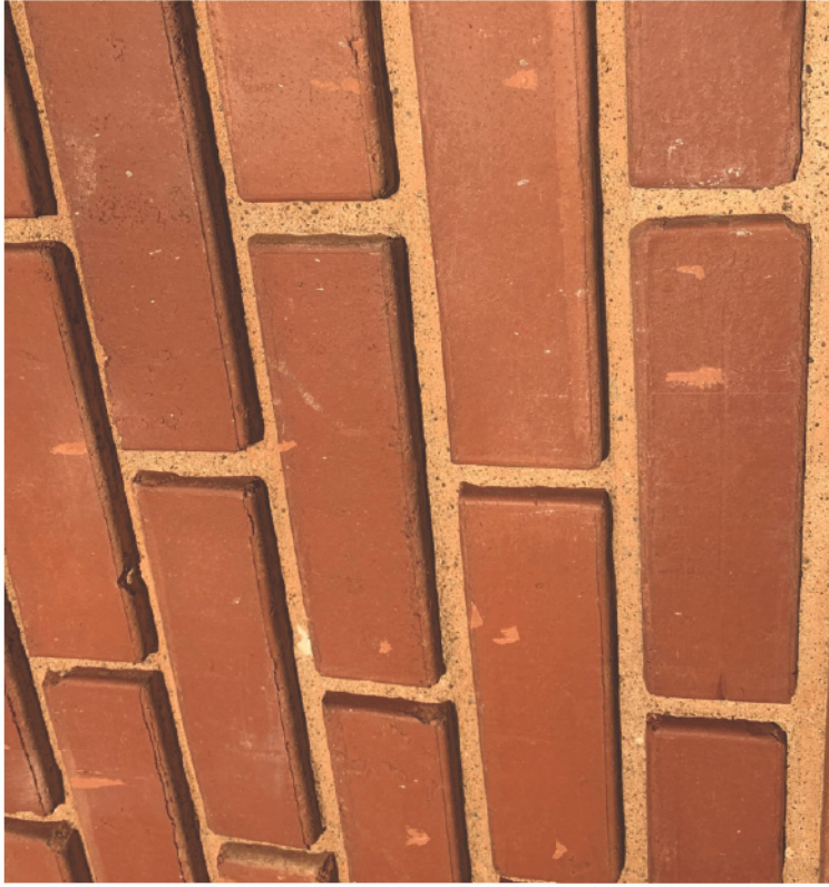
EXISTING 8 5/8" X 4" X 2 1/2" SOLID BRICK- NEW BRICK AND GROUT TO MATCH EXISTING IN COLOR AND TEXTURE
