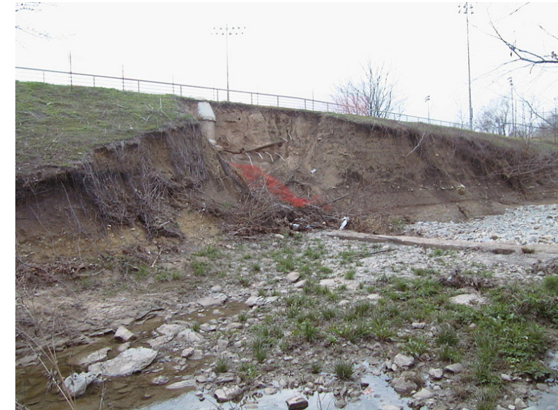
Stream erosion threatening wastewater infrastructure
