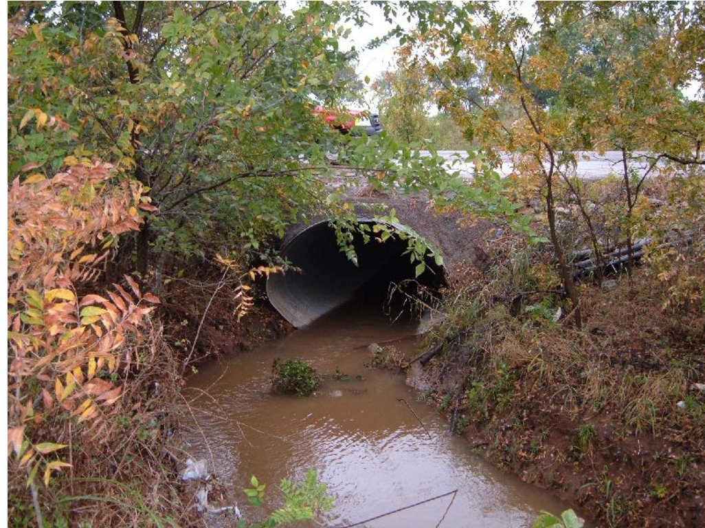
Culvert view downstream side of Franklin Road – Trib. G to Little River
