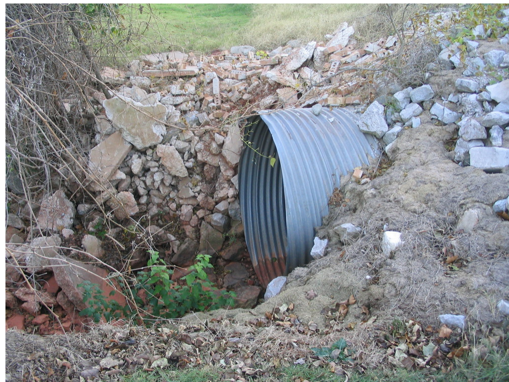
No culvert headwall downstream of 36th Street NE – Rock Creek
