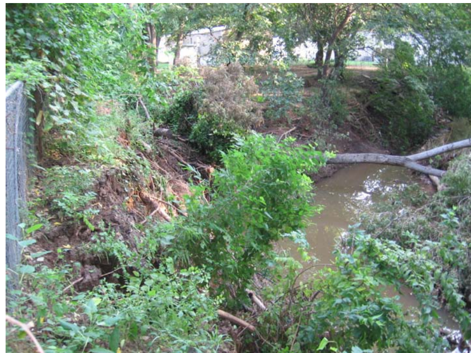
Stream erosion downstream of Main Street – Brookhaven Creek
