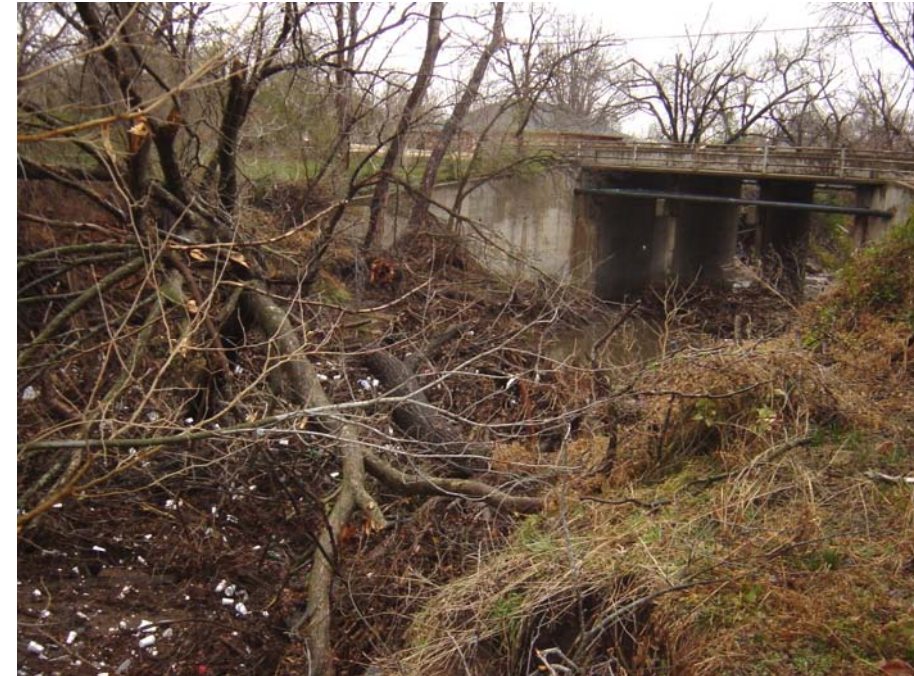
Debris blocking Imhoff Creek
