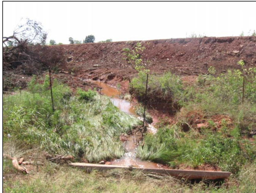
Downstream side of unmaintained dam
