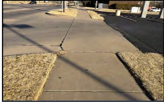
Corner 4 No Ramp (4z)
