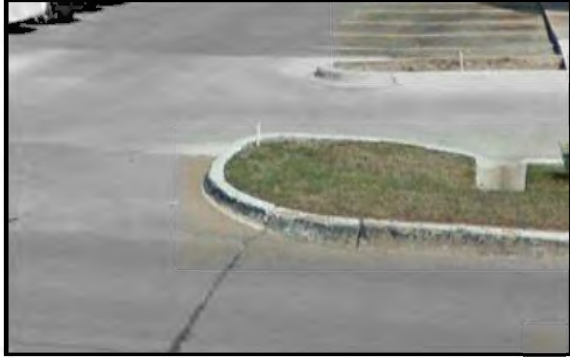
Corner 3 No Ramp (3z)
