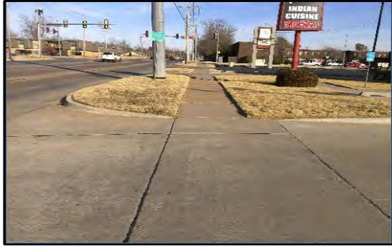
Corner 3 No Ramp (3z)
