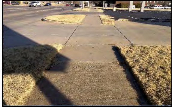
Corner 4 No Ramp (4z)
