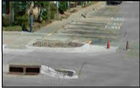
Corner 2 No Ramp (2z)
