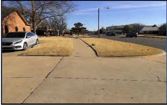
Corner 3 No Ramp (3z)
