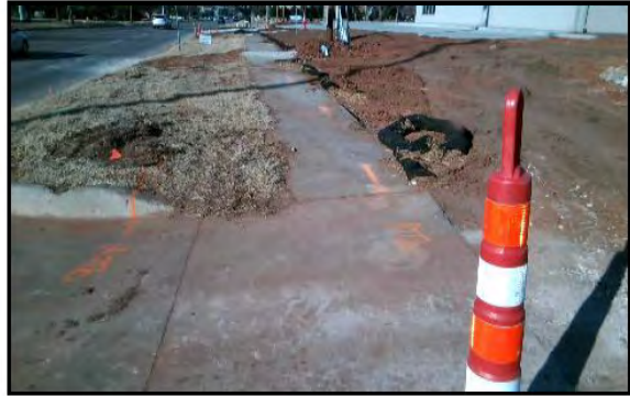
Corner 2 No Ramp (2z)
