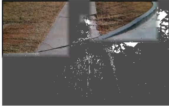
Corner 2 No Ramp (2z)
