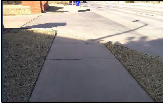
Corner 3 No Ramp (3z)
