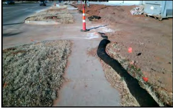
Corner 3 No Ramp (3z)
