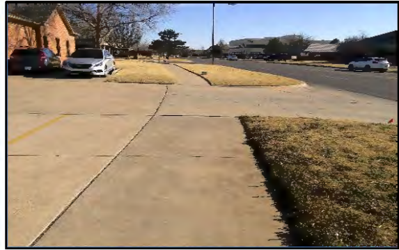
Corner 2 No Ramp (2z)
