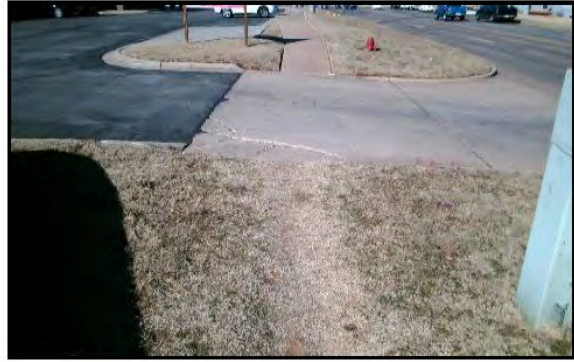
Corner 4 No Ramp (4z)
