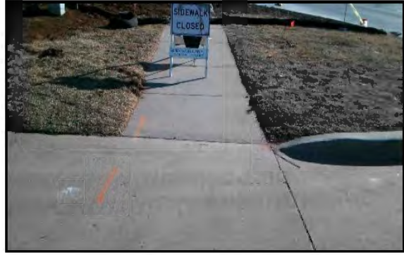
Corner 3 No Ramp (3z)
