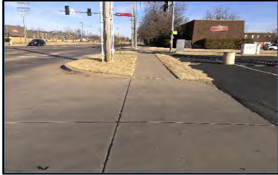
Corner 3 No Ramp (3z)
