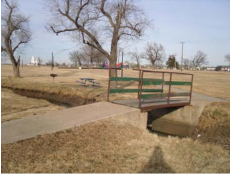
Though functional, this pedestrian bridge in Frances Cate Park is just barely accessible and is not an attractive feature of the park.
