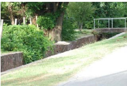
The WPA drainage channel is a significant historic feature in the neighborhood but some consider its condition a liability.
