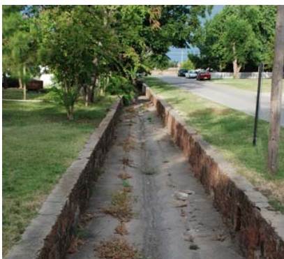
The stone-lined channel of Imhoff Creek was built by the WPA during the 1930s.
