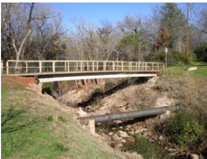
The pedestrian bridge over Bishop Creek in Eastwood Park represents a future opportunity for a highly functional placemaking element.
